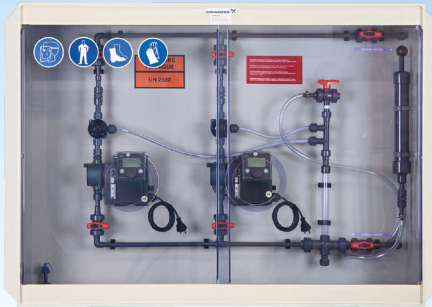
Dosing cabinet skid
